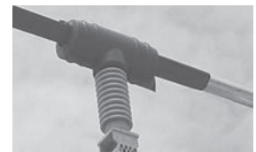
2 MVLC-38 on busbar with BCIC
