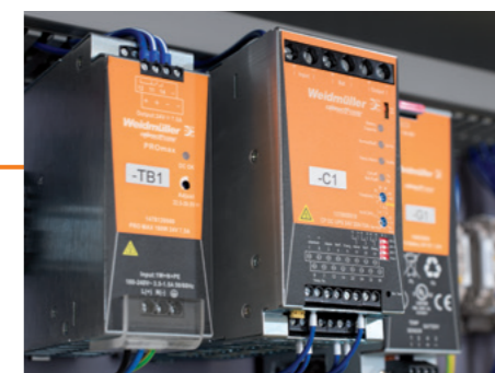
ESG: All-purpose equipment identification – simple labelling of markers for quick identification of components
